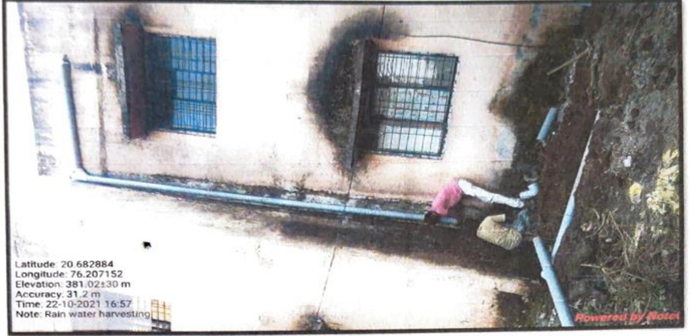
7.2/ 3: PVC Pipes System For Roof Top Water Harvesting.
