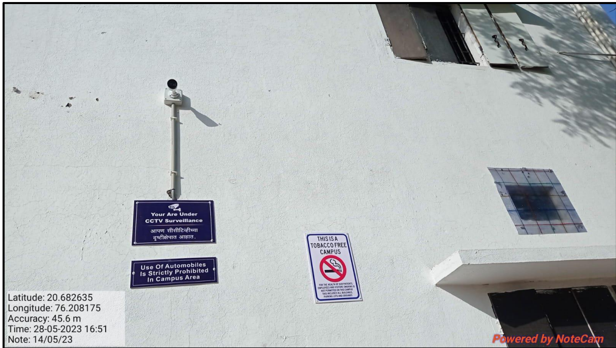
Photos of CCTV Surveillance in College Campus
