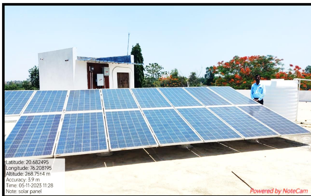
Solar Panel of 5 KW
